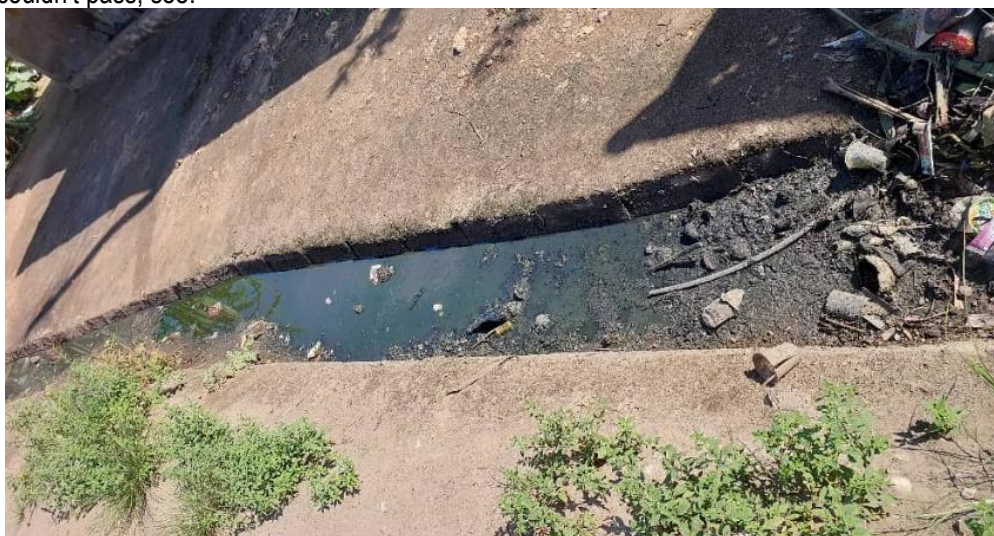
Figure 4-9: Condition of some of the existing drainage systems along the proposed roads in the DCC
