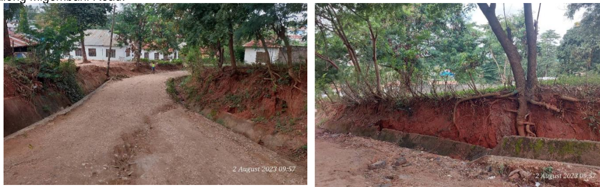
Figure 4-10: Erosion of the roadsides along the Migombani road
