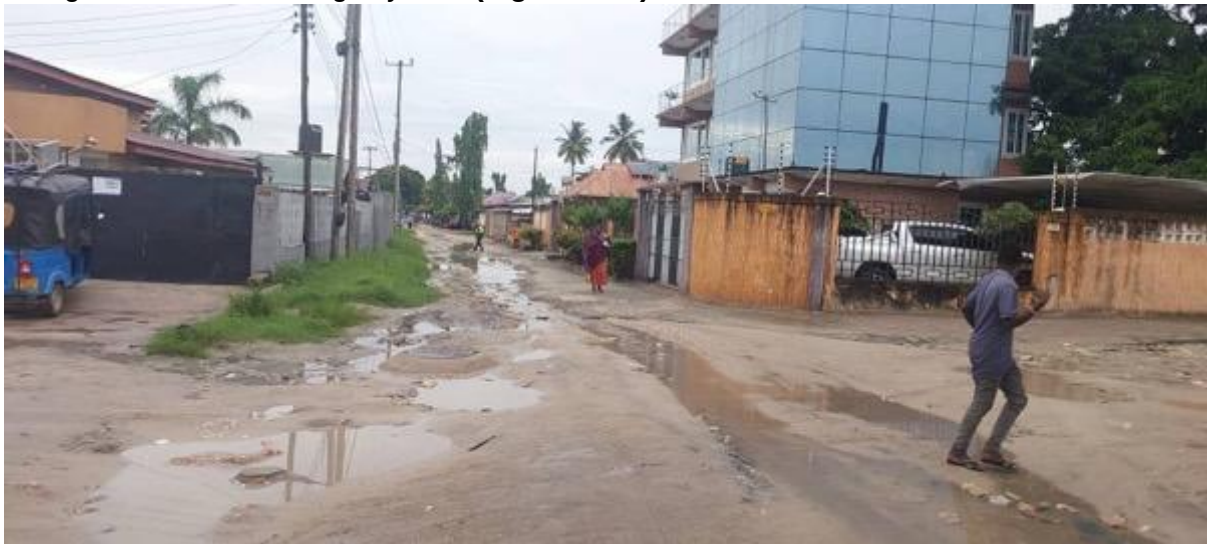
Figure 2-79: Water Ponding Problem at Segesera Road, Photo Taken at 0+300
