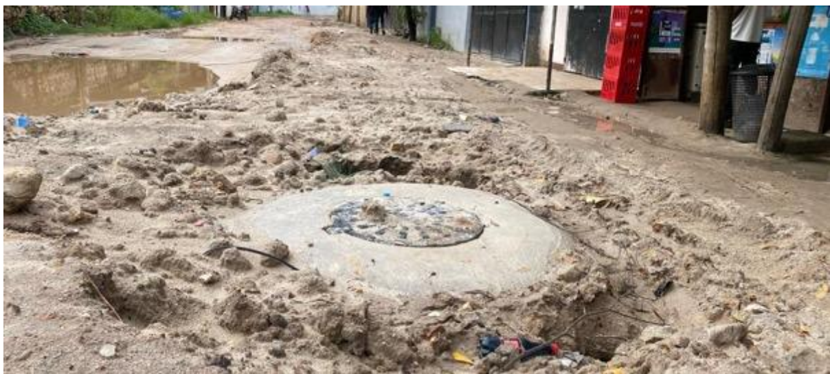
Figure 2-55: Standing Water and Sewer Manhole at Sheikh Bofu Road, Photo Taken at Km 0+200
