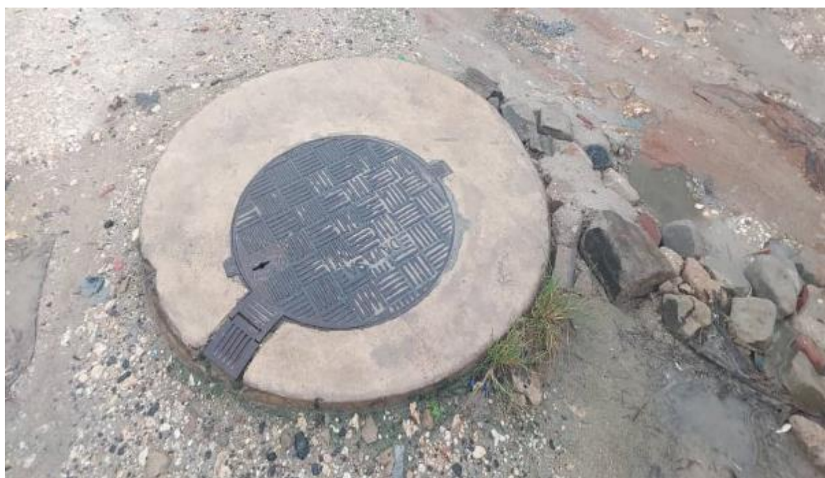
Figure 2-94: One of Sewer Manholes found at Km 0+800 of Juma Ikangaa Road
