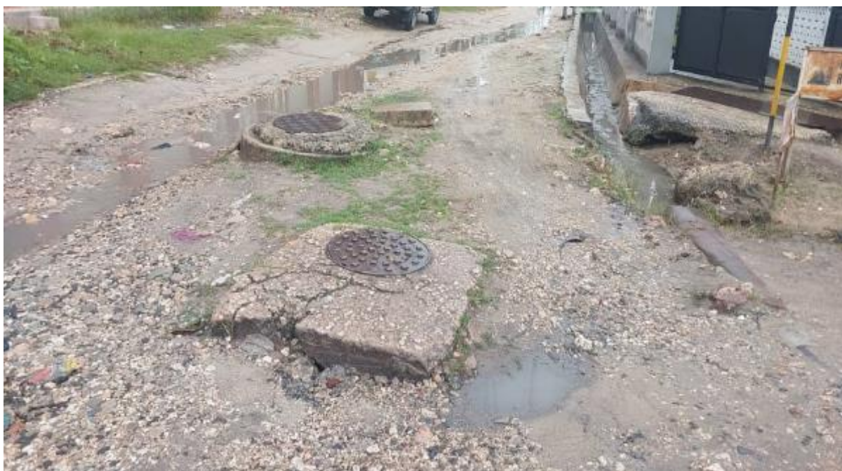
Figure 2-87: Manholes for Sewerage System at Km 0+210 RHS of Segesera Road
