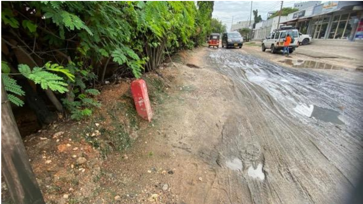
Figure 2-62: Concrete Marker Post of Airtel Communication Cable Km 0+000 LHS, Sheikh Bofu Road
