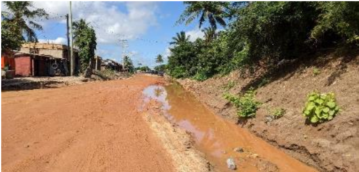
Figure 2-34: View of Goba – Wakorea Road at Km 2+350 Side Drains/Ponding Problem
