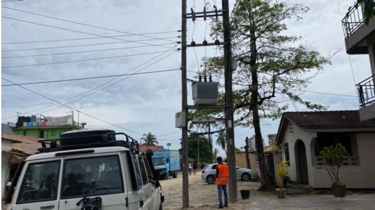
Figure 2-60: 13kV Electric Power Substation at 0+700 RHS of Sheikh Bofu Road
