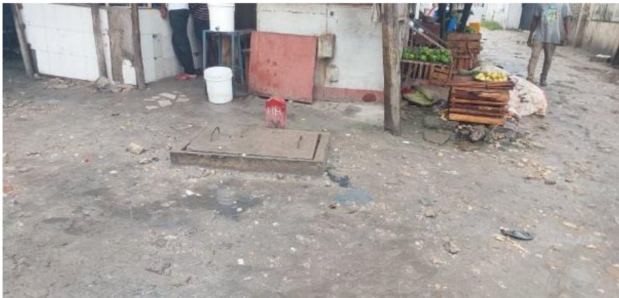
Figure 2-86: A Manhole for Halotel Telecommunication Cable at Km 0+050 LHS of Segesera Road
