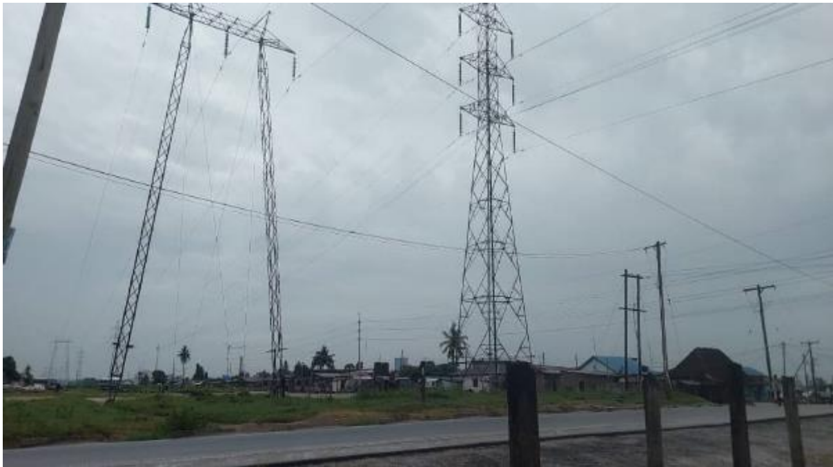
Figure 2-149: High Tension Power Line Crossing the Existing Tarmac Road at Km 0+100
